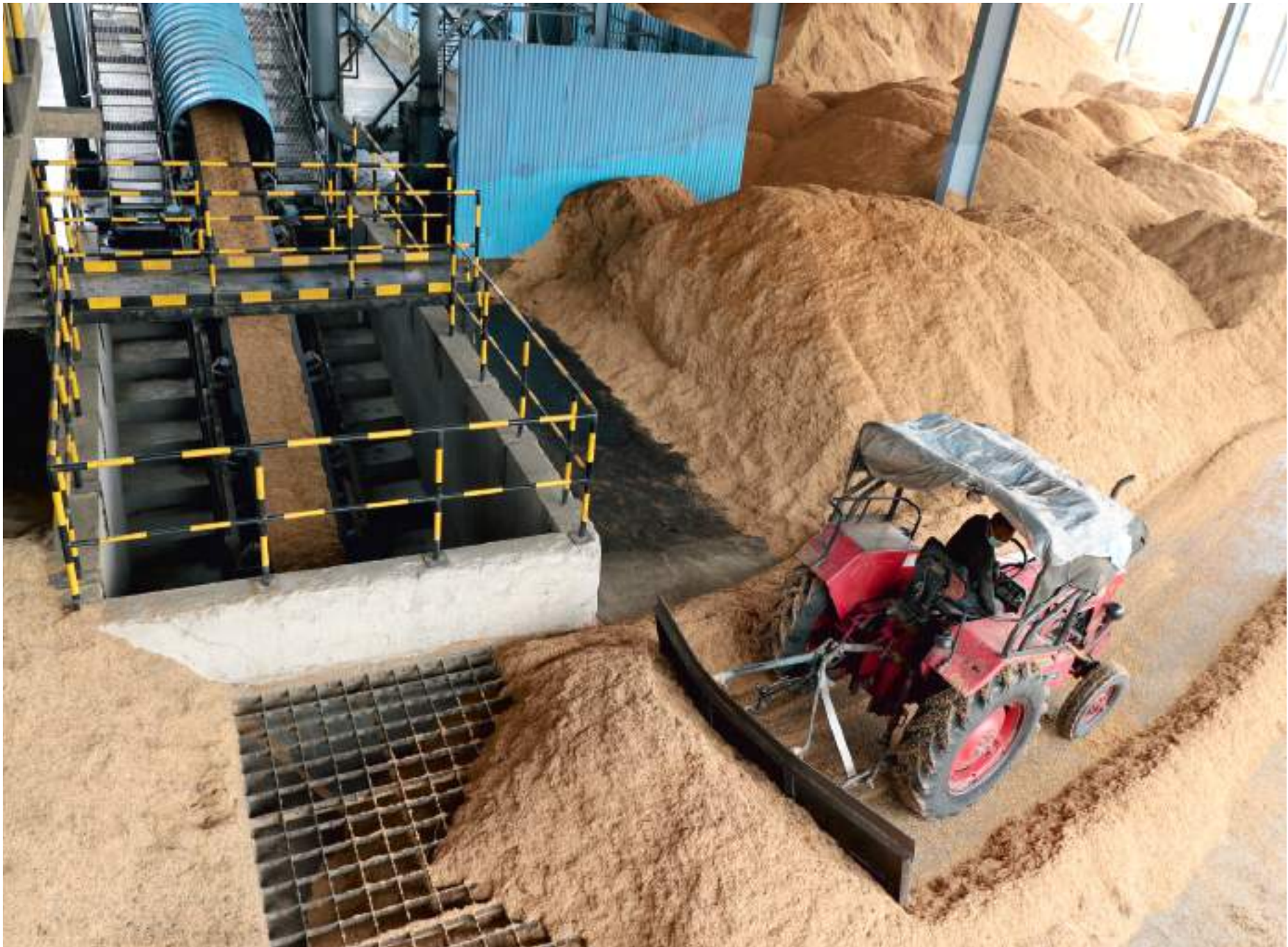
Utilisation of husk as fuel in power plant boiler to reduce coal usage
