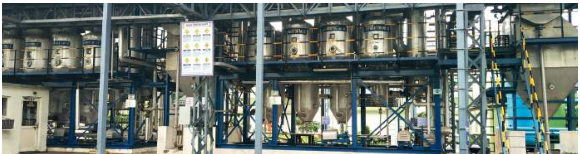
Caustic Recovery Plant
