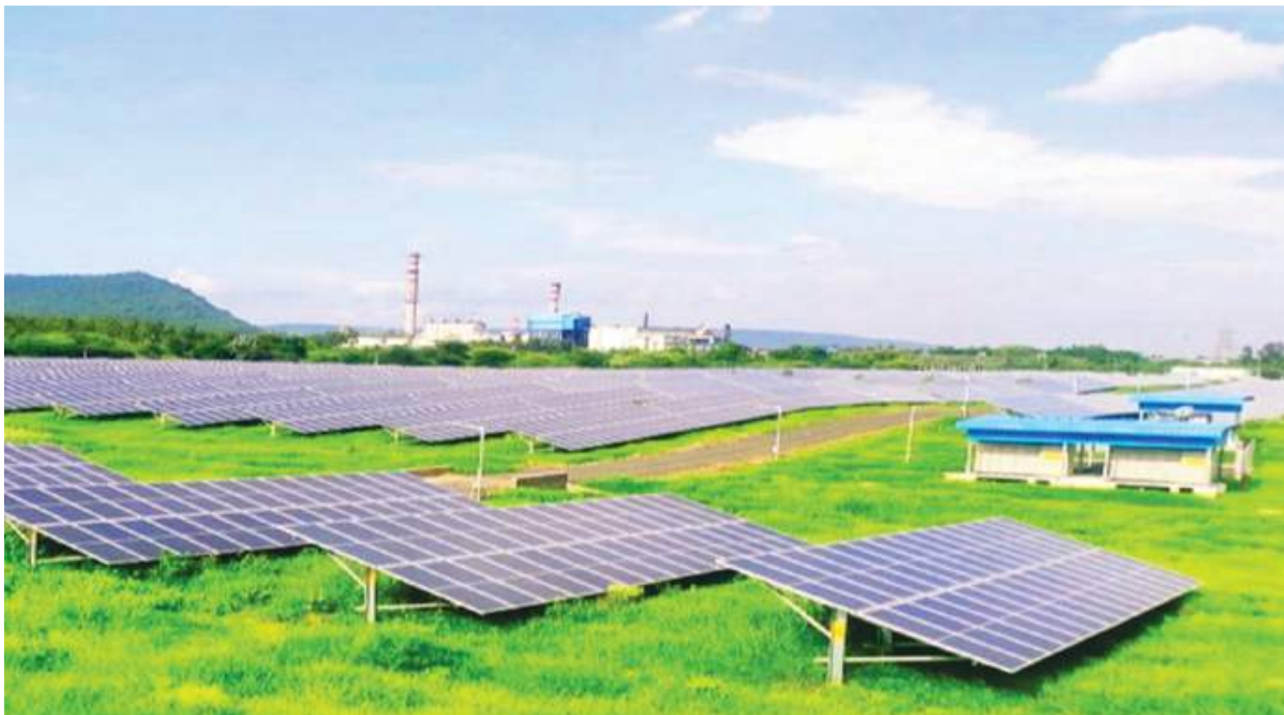
■ Ground Mounted Solar Plant, Vardhman Fabrics, Budhni
