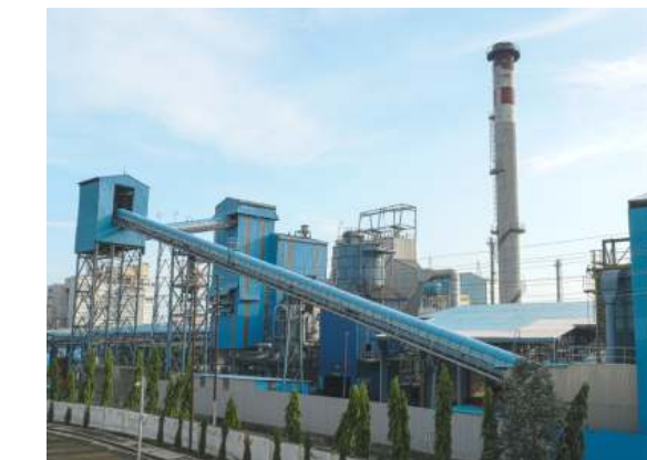
40 TPH Boiler, Baddi
