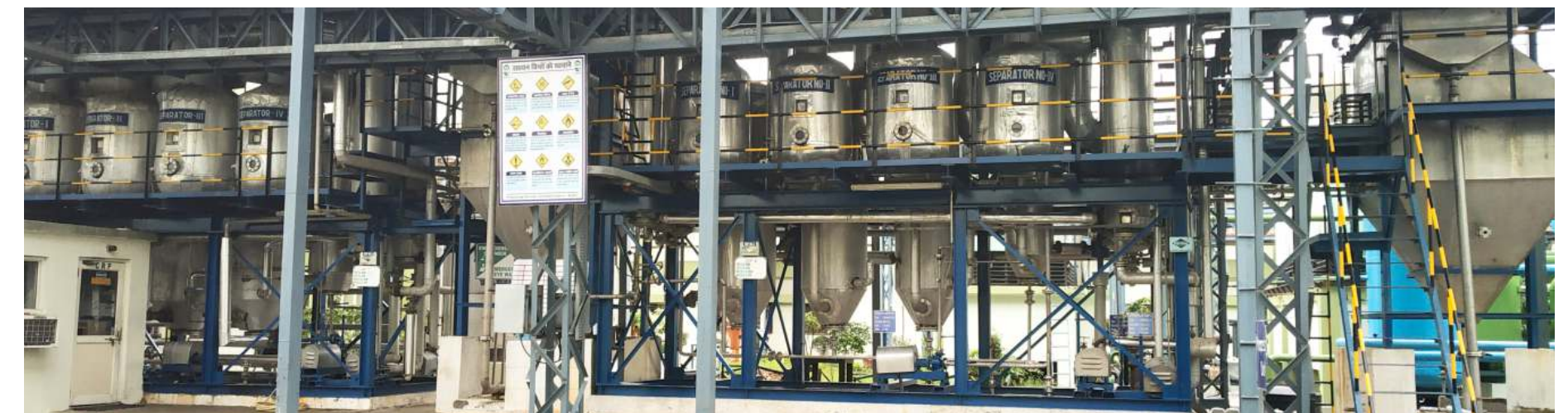
Caustic Recovery Plant
