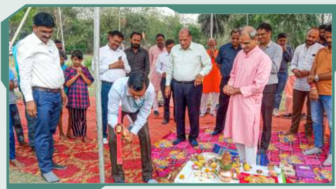
The foundation laying ceremony for the construction of two classrooms, an Anganwadi Bhawan and a toilet facility at Government Primary School, Mandehri, Mandideep District, Raisen, Madhya Pradesh
